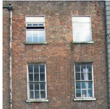
Brick Damage- Rutland Street
