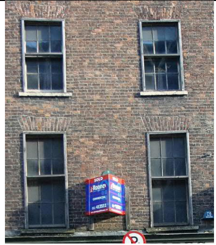
Brick Damage – 4 Patrick Street
